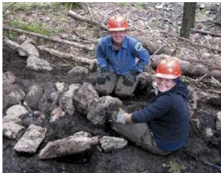
The Maine Conservation Corps crew members set stones on a section of the Osgood Trail to harden the walking surface.
